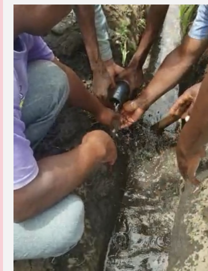
In Samaria, Tanzania, villagers are working Mondays, Wednesdays, and Thursdays to dig the trench for the pipeline to Savana Primary School. In addition to bringing water to the 400 students at the school, the 9 km pipeline will also provide water to Zaire and Savana villages, with a total of six water stations. There will be over 3000 people who now have access to water thanks to this project. Asante sana!
